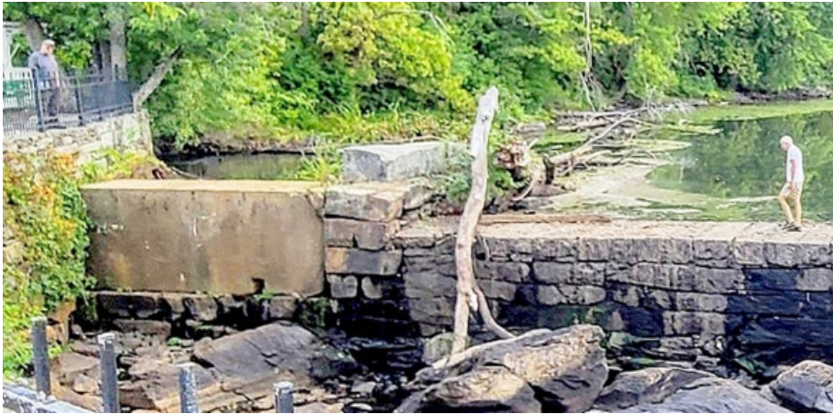
Entrance to 1828 fishway blocked by concrete.
