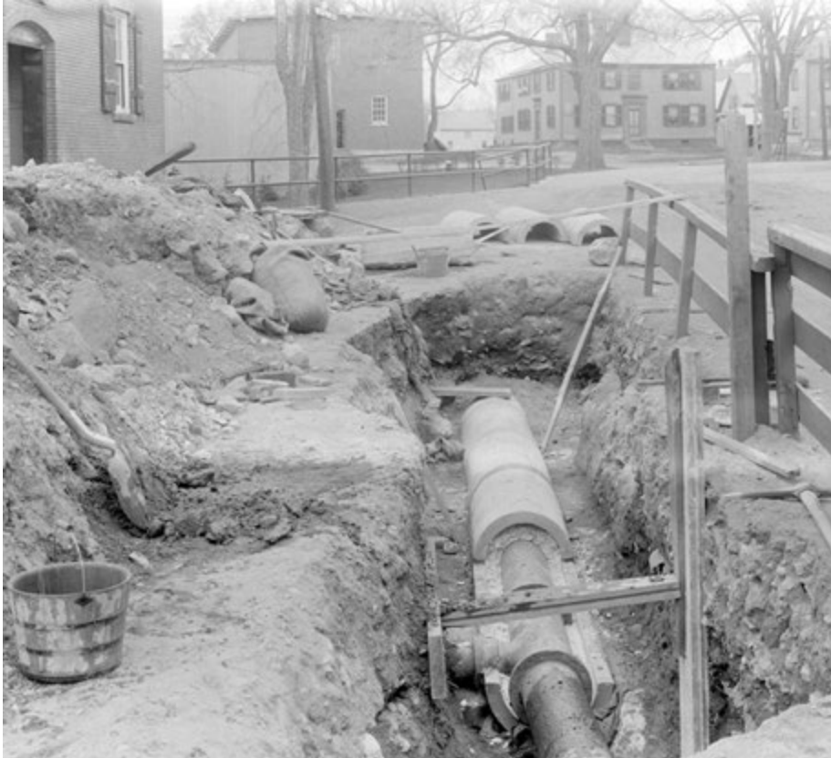
Water main project showing the corner of 2 Old Elm Street. the warehouse at the end of the museum parking lot, the Joel Dix (Canal Boat Captain) House and a piece of the Middlesex Hall which was an extension of the Mears Tavern
